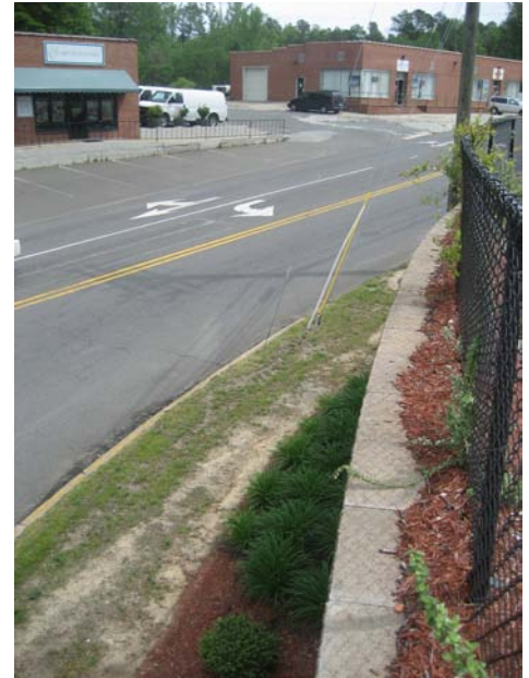
A worn footpath along the retaining wall at the intersection of NC 50 (Main St.) and NC 56.
